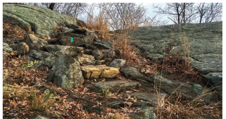
The Long Distance Trails Crew built this beautiful staircase on the new Long Path reroute.
